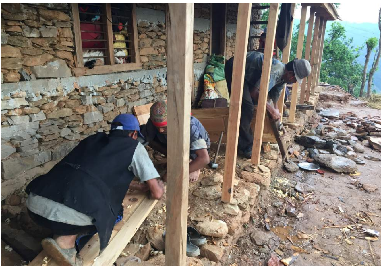
Photo: Luisa Miranda Morel, 2017. 'Working on other people's houses is good so they will come and help me build mine' – rebuilding in Nepal
