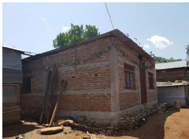
Figure 13: Load-bearing brick walls with cement mortar and reinforced concrete corner posts and bands
