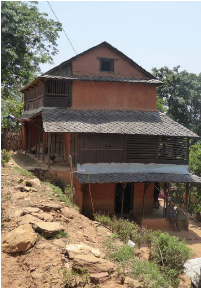
Figure 9: Traditional house in Dhading with three storeys plus attic, load-bearing masonry walls and timber floors and roofs, with external timber verandas
