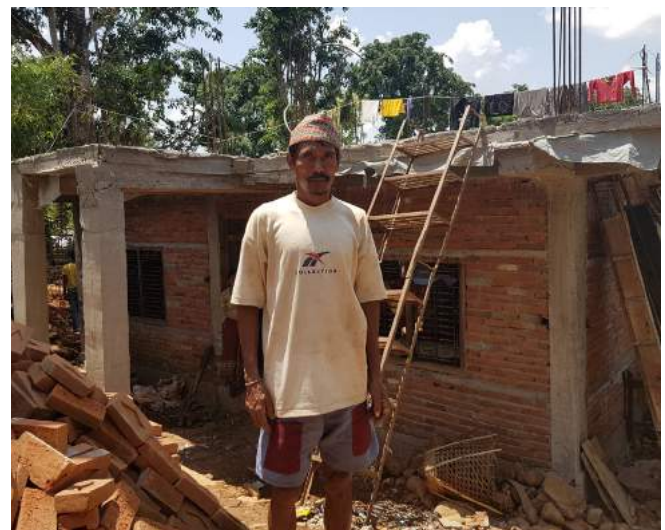
Figure 11: Reinforced concrete frame with brick infill, one storey with reinforcement bars at all columns ready to build a second storey in the future
