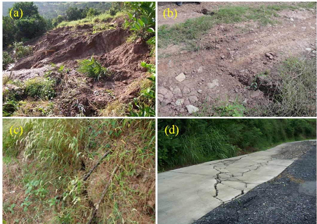
Figure 5. The deformation phenomena on the landslide mass: (a) slump of TH1, (b) crack of L2, (c) crack of L4, and (d) crack of L9.
