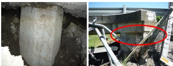
(c) Cracking at the top of the abutment piles (d) Cracking of the abutment-deck connection
