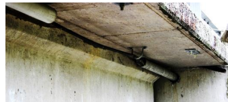
(c) Telecom line (Lower Mason Bridge)
