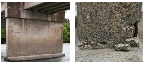
(e) Cracking and buckling at the base of pier
