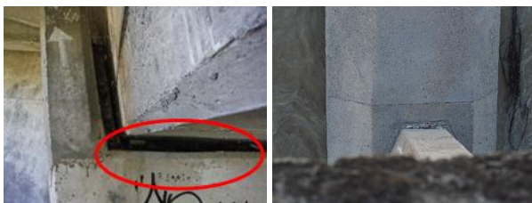
(c) Deck settlement (d) Concrete spalling at pier base
