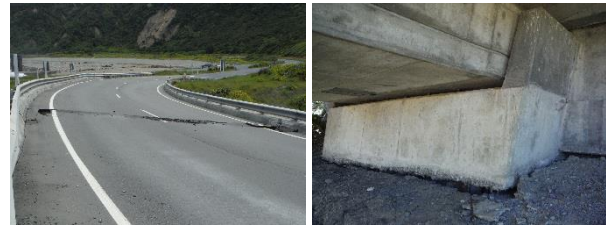
(a) Approach settlement (Mororimu Stream) (b) Abutment fill settlement (Clarence River)
