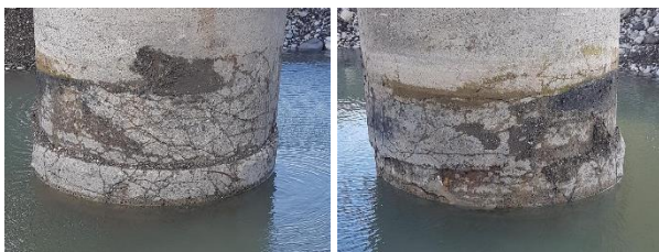
Figure 33: Typical pier damage observed after excavation and dewatering [courtesy of OPUS International Ltd].
