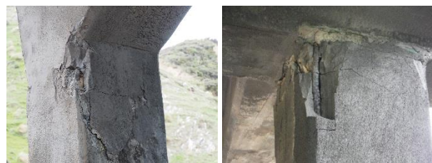
(c) Cracking below knee joint of central pier (d) Close up of exposed bar at the top of a column
