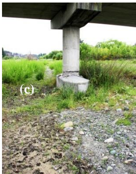
(c) Liquefaction ejecta near central pier. (Mason River Bridge)
