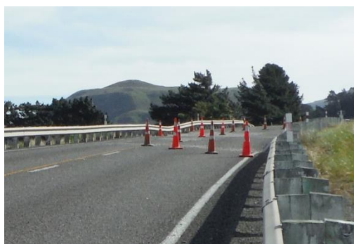
Figure 39: Fill settlement and spread at the Waima Overbridge.
