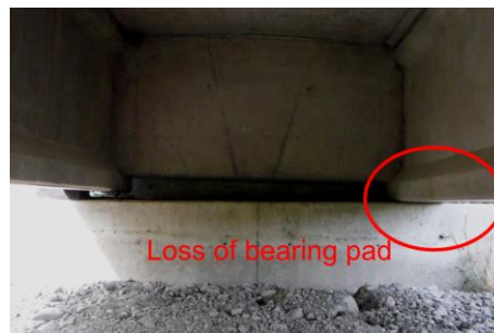
(b) Residual displacement of bearing (left in image), unseating from elastomeric bearing (right in image)
