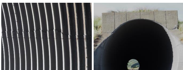
(c) Cracked surface coating at flattened part of the arch lining (d) Cracking of concrete surround at the southern end lining
