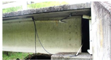
(a) Telecom cable (Hanmer River Bridge)
