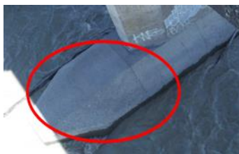
(e) Damaged pile cap
