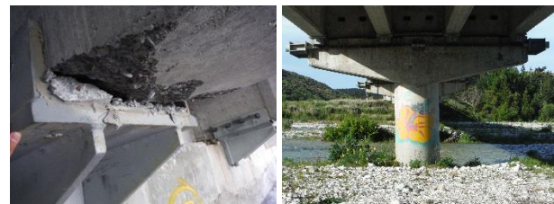
(c) Spalling of concrete around the retrofitted steel brackets attached to the beams (d) Slight tilting of the first pier from the southern abutment westward
