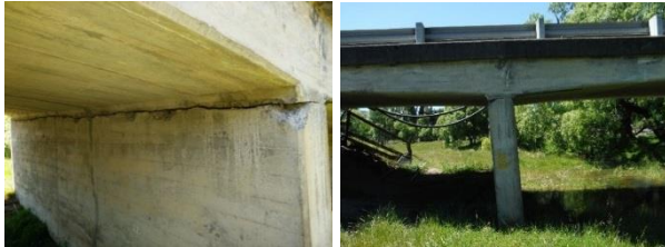
(a) Typical cracking at the top of the piers (b) Tilted pier
