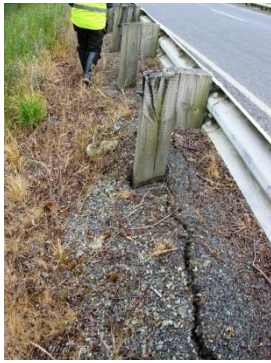
(a) Embankment failure due to lateral spreading (Hanmer River Bridge)
