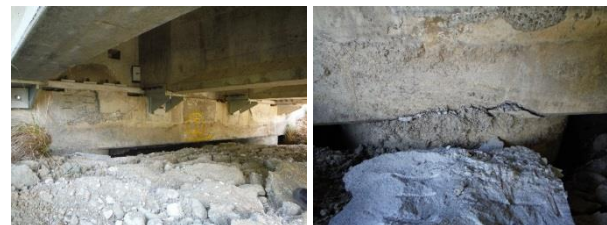
(a) View of the south abutment (b) Cracking of the pile – abutment interface
