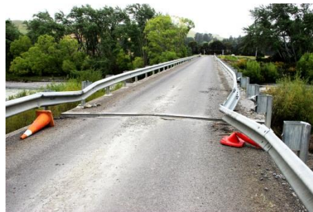
(a) Compression failure of the expansion joint over the central pier
