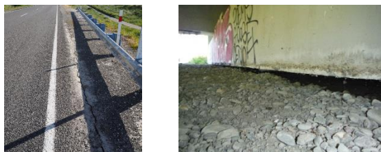
(c) Lateral spread crack at bridge approach (d) Settlement of abutment fill
