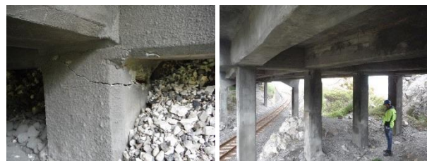
(a) Abutment column cracking (b) Spalling at the top of the column bent
