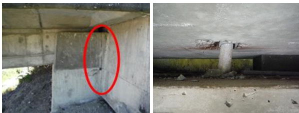
(a) Abutment cracking (b) Hold down rod residual deformation
