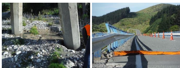
(a) Liquefaction ejecta (b) Large approach settlement (Orange spray paint)
