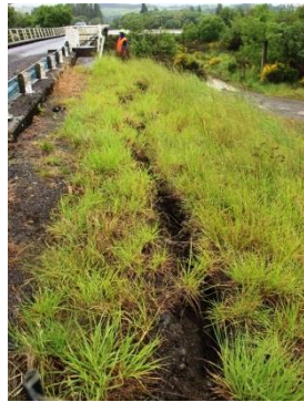
(b) Embankment failure due to lateral spreading (Waiau River Bridge)
