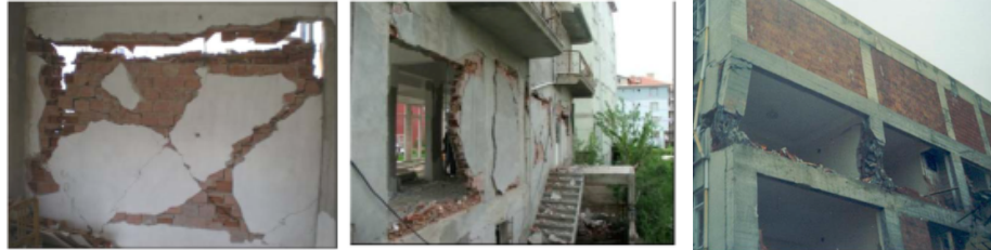
Figure 3. Typical out-of-plane failure of URM infills in RC framed building, showing top-down collapse creating new voids that reveal the underside of the RC beams.
