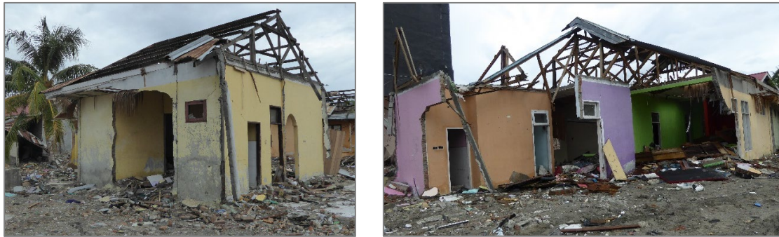
Figure 10. Heavily damaged CM houses in Palu bay area along the Jl. Rajamoili road, about 100m from coastline. The walls of this house were directly hit by the tsunami inundation.
