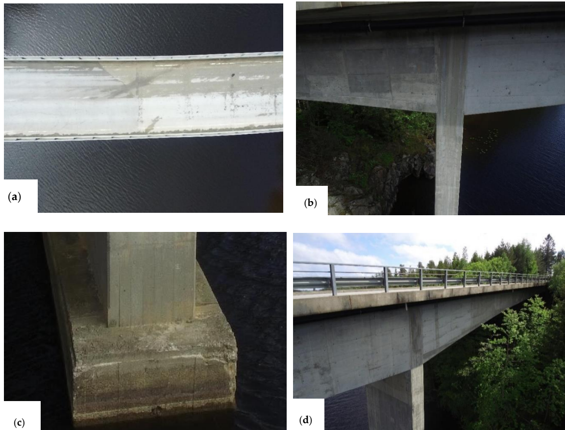
Figure 4. (a) Top view of Skodsberg bridge. (b) drone image of detail near top deck and footing. (c) drone image of concrete deterioration. (d) Unmanned Aerial Vehicle (UAV) photo detail near the top deck and footing.
