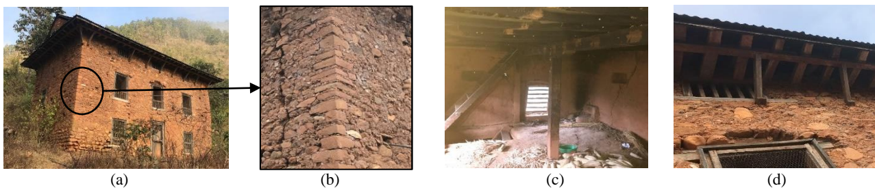
Fig. 1 – Construction characteristics of a typical PRE- SMM building: (a) 3-D view, (b) view of a corner connection, (c) longitudinal timber frame and floor structure, and (d) timber roof system with timber keys and compression struts
