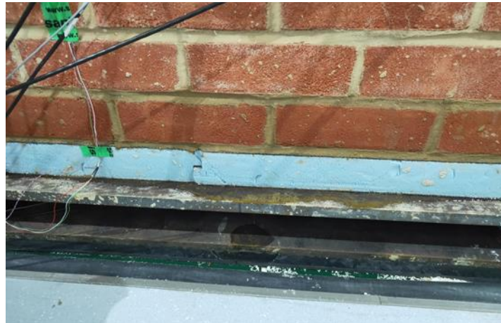
Figure 7: Example of water penetration to the interior surface of the interior leaf
