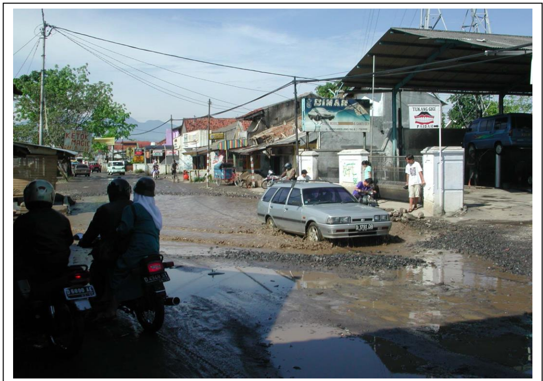
Figure 5.24 The absence of collective road improvements at the northern gate of the MRRA. The road quality was so poor because of the absence of a proper drainage system. Rainwater and traffic had contributed to the severe damage of the road construction. Residents seemed more concerned about the improvement of infrastructure in their neighbourhood that was needed more immediately. Source: field survey 2002.
