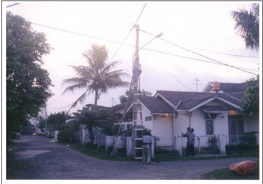
Figure 5.30 An example of street lighting installation. Public street lighting was only available in the main public area, which was in the surroundings of a shopping centre. Most of the road network in the area was in total darkness, unless residents installed lighting. The picture shows the work of a community that decided to install street lighting of a good standard. It was common for residents to install a simple street light (a lamppost), such as the one standing in front of the house. That was actually a result of previous mutual-self help project to install uniform simple street lighting in each house plot. Source: field survey 2002.
