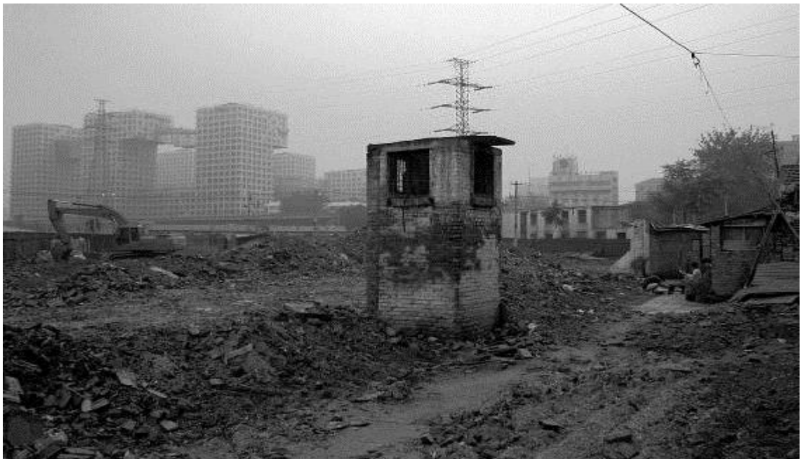
Figure 53: Demolition of the workers' community with linked Hybrid in the background. (Photo Cressica Brazier, 14 June, 2008).
