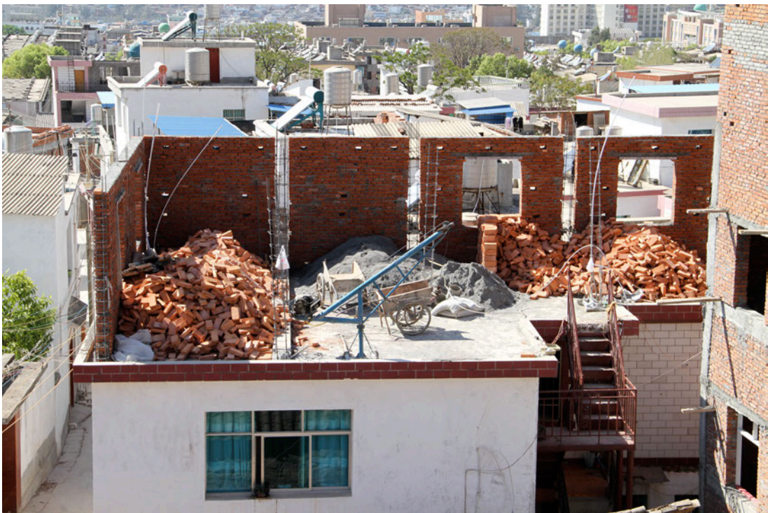
Figure 9: Wall on village-in-the-city home. Steel mesh uprights are visible in spaces in-between wall.
