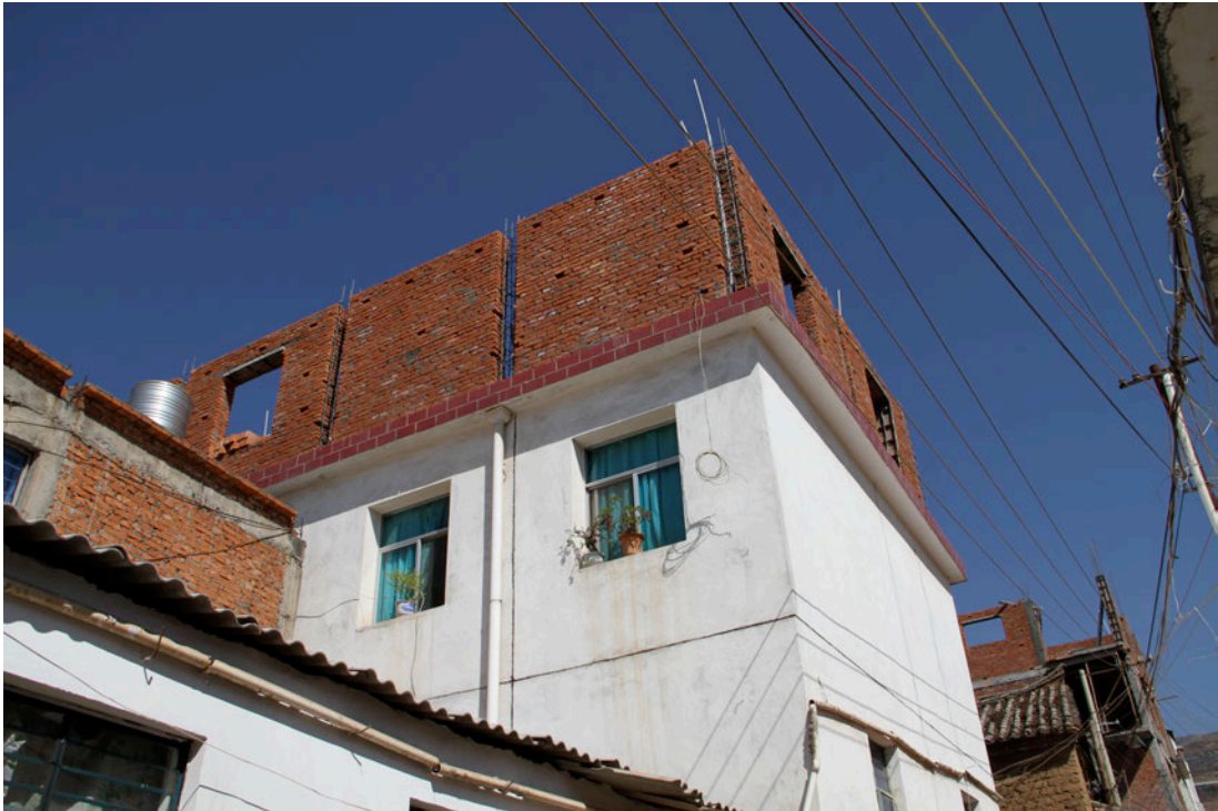
Figure 12: Adding an extra floor on top of an existing village-in-the-city home prior to new building regulations coming into force
