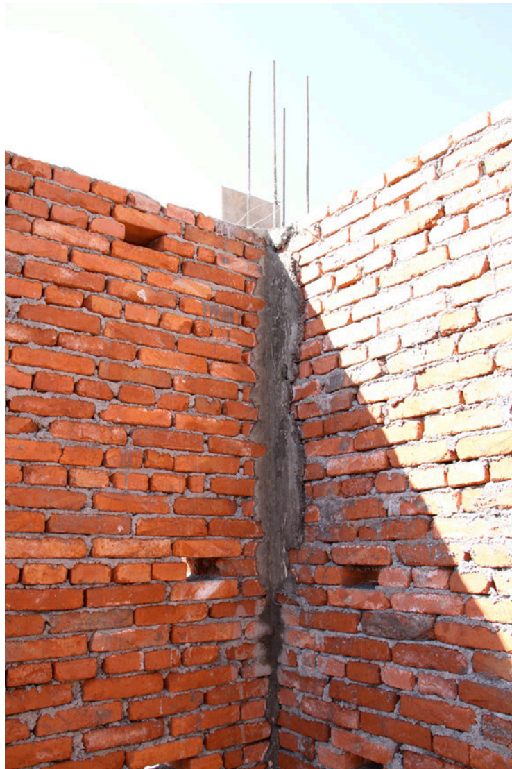
Figure 10: Steel mesh left sticking out of top of column in village-in-the-city home to allow for future expansion
