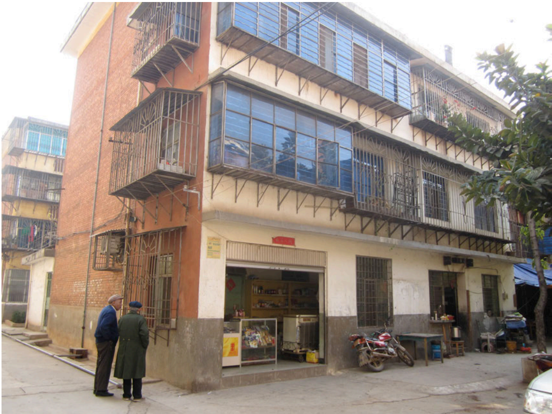
Figure 15: Unsanctioned expansion of an early work-unit block of apartments. The concrete-faced brick section of building with windows has been added on to the original exposed brick work-unit apartment block behind it.
