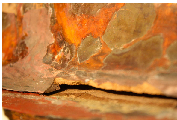
Figure 5 Detail of the area where the old repairs that attached the sculpture to the pedestal had failed. Image: ©Hsinhui Hsu.
