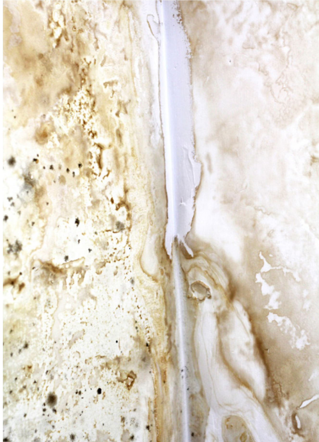
Roithmayr, Florian (2015) water damaged wall , photograph taken of the PhD room, Slade School of Fine Art, UCL.
