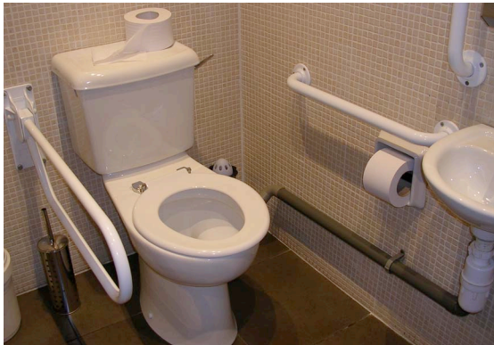
Figure 6: Flush handle fitted on wrong side of WC pan Photo; VivaCity 2020: 2005
