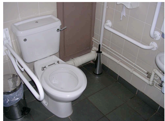
Figure 5: WC pan placed too far from the wall. Photo; VivaCity 2020: 2005
