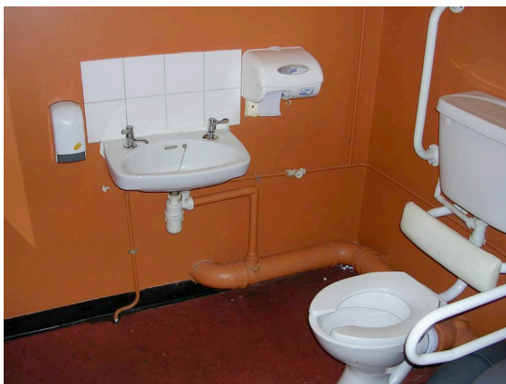
Figure 4: Washbasin fixed to opposite wall, drop down rail fixed on the wrong side of WC pan.
