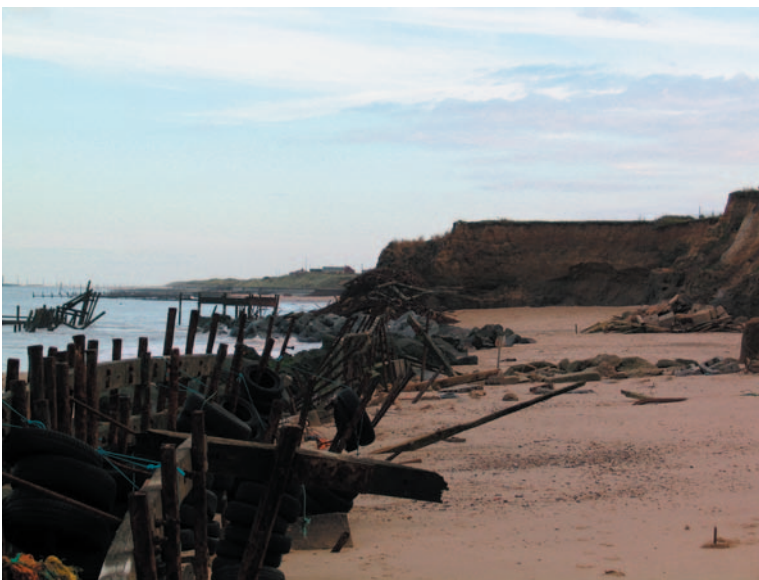
Images 4-6 Eroded revetment and cliffs produce a new landscape on the beach.
