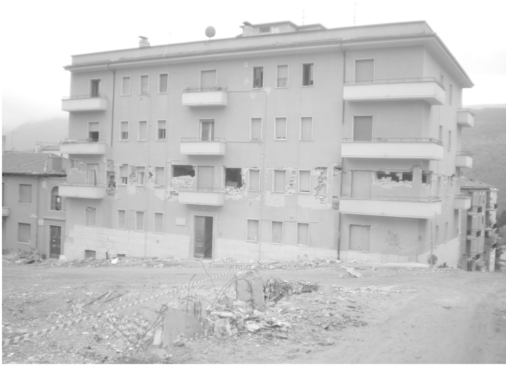
Figure 2. An example of incipient mid-floor failure in L'Aquila city (photo: author).
