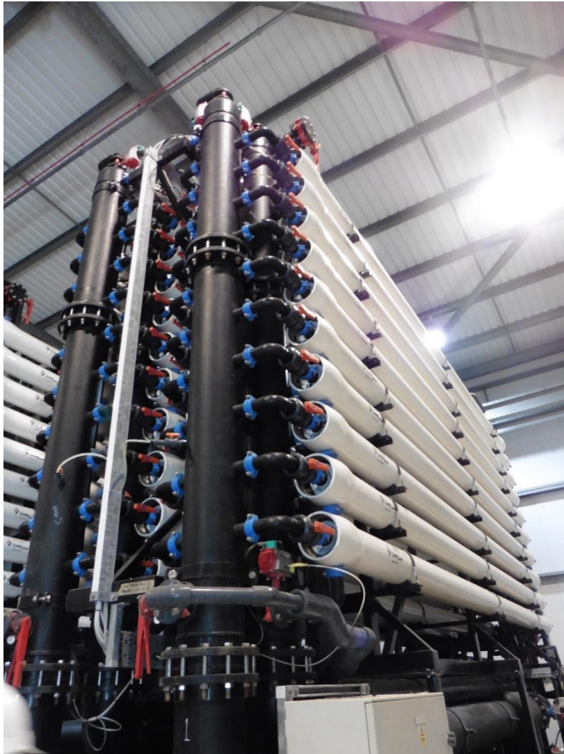
Figure 15: Reverse osmosis filters at the Beckton desalination plant, London. Source: Fieldwork photo.
