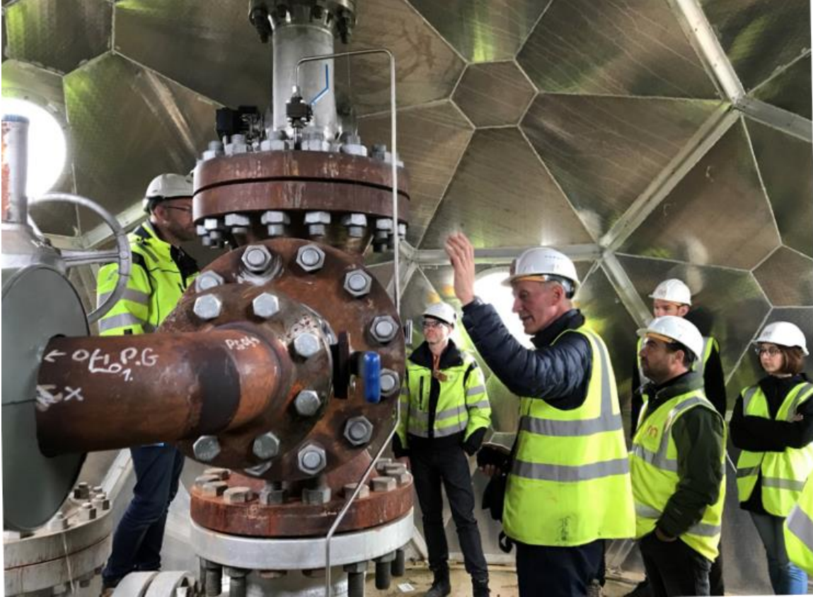
Figure 6. Siggi explaining the CarbFix CO 2 -H 2 S injection system, June 2016.
