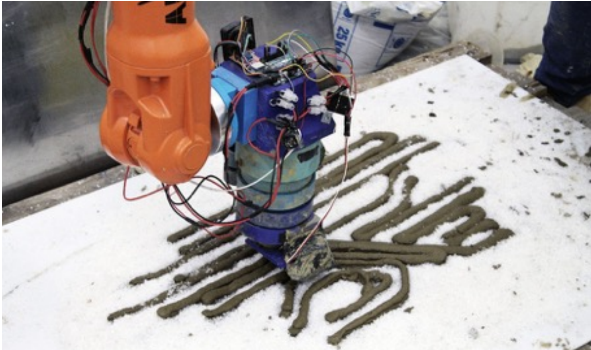
Robotic Concrete 3D printing – RC4 204-15 // Team Amalgama: Francesca Camilleri, Nadia Doukhi, Alvaro Lopez Rodriguez and Roman Strukov
