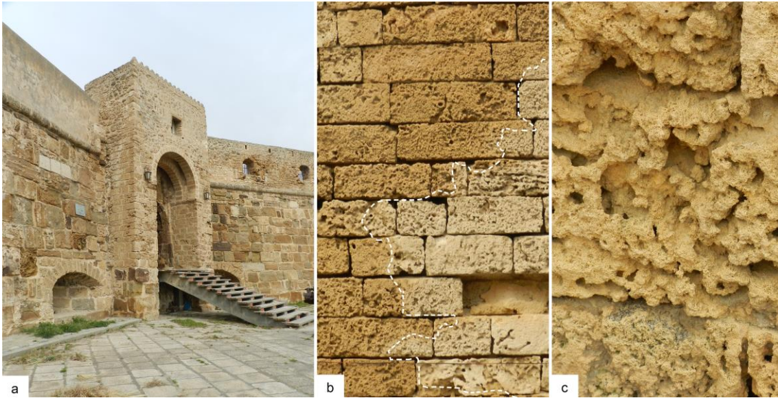
Figure 1. a) Spanish Fort of Bizerta (view from the port); b) Wall of the Fort with honeycomb weathering and moisture problems; c) Honeycomb weathering and loss of material on decayed stone ashlar
