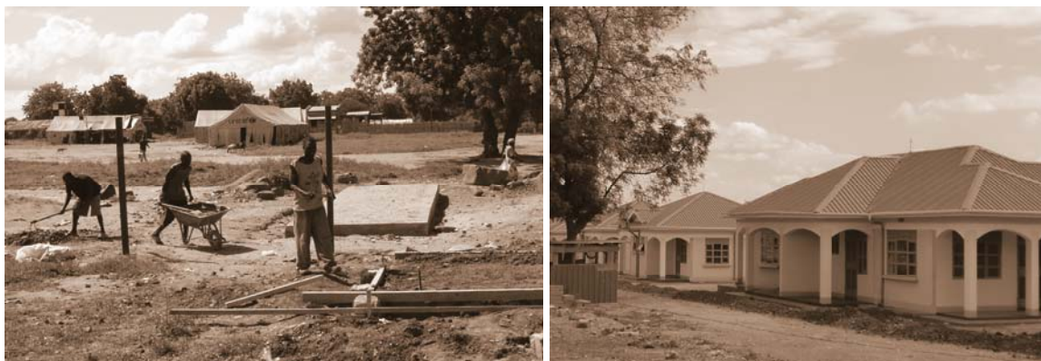
Juba Technical, then and now. Plan hopes that this will be the standard for reconstruction of TVET facilities in South Sudan. Left, building the perimeter fence. c. Berkeley Hackett, November 2006. Right, the new teachers houses. c. Ndūng'ū Kahīhu, December 2009.
