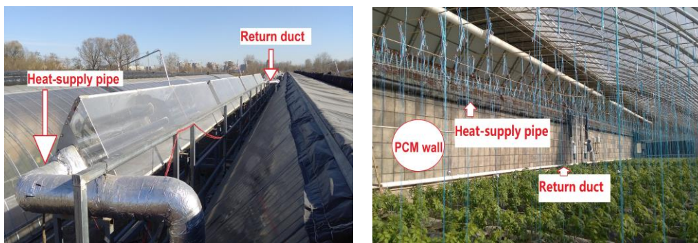
Fig. 21 The appearance of the installed MSC-DRTs and interior of the experimental solar greenhouse.
