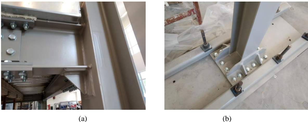
Fig. 2 – Locations of stiffeners: (a) at beam column connection and (b) at column base
