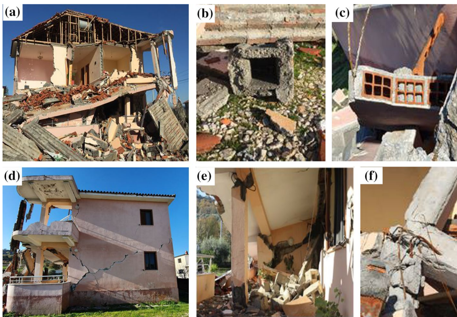
Fig. 9 Single-family rural houses in Bubq. a Failure of the front part of the building due to the collapse of the portico porch, b hollow concrete blocks of the bearing walls, c detailing of the hollow core prefabricated concrete slab, d severe crack of the rear building's façade due to the failure of the portico porch, e internal view of the portico porch, f details of the joint failure due to poor smooth reinforcements, which are completely corroded
