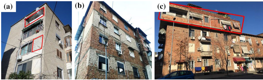
Fig. 19 Unauthorised interventions on unreinforced masonry (URM) buildings in Durrës. a Irregularities in the opening layout due the closure of part of the balcony; b use of different construction materials and c presence of an additional floor
