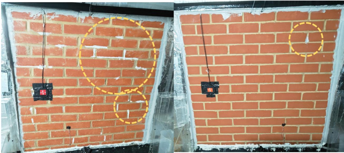
Figure 18 Sample of defects observed in the mortar joints of the walls tested (in the picture walls C1 and A2) .
