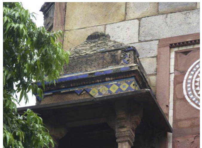
Fig. 2. Glazed tiles employed on a jharokha , an ornamental architectural feature, on Arab-ki-Sarai Gate.
