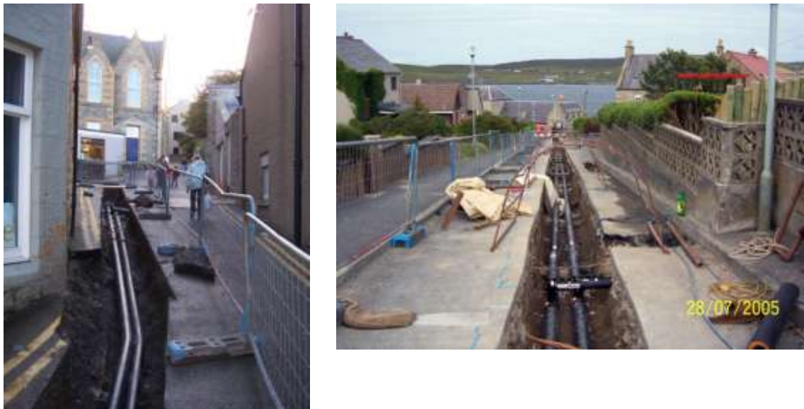
Figure 18: Photographs of heating pipe installation in Lerwick (Shetland Heat Energy and Power Limited, 2011)
