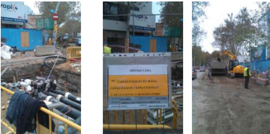
Figure 7: Photos of Districlima pipe installation, Barcelona (Cary, [Photographs of Districlima pipe installation], 2012)
