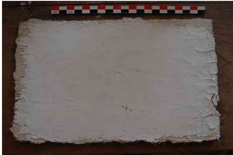
Fig.142 The second (finer) white marl plaster layer without straw, applied onto the first layer.
