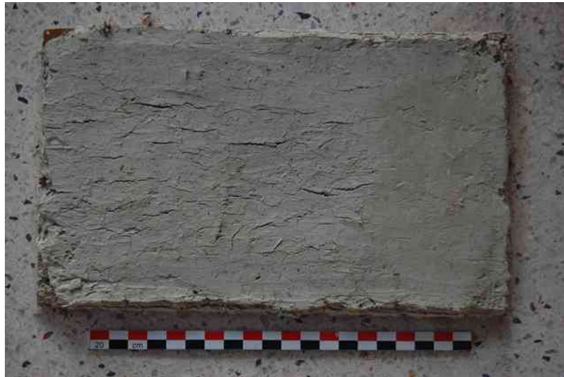
Fig.145 Marl plaster layers cracking during the drying process.
