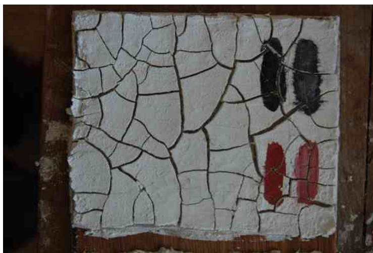
Fig.153 Wet marl plaster cracking upon drying.
