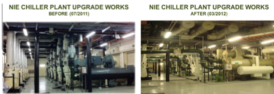
Figure 2. The HE campus plant room before and after upgrade.
