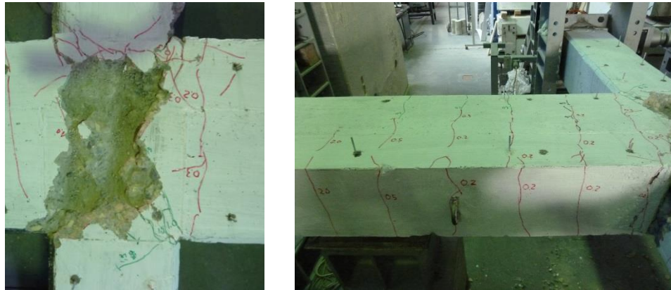
Fig. 4. Final damage state in C-noSLT; left: joint, right: beam
