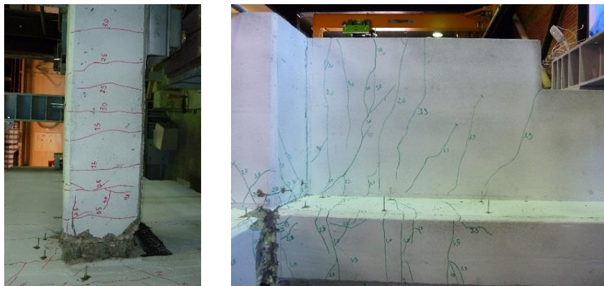
Fig. 8. Final damage state in C-EC8; left: superior column, right: beam underside
